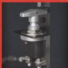
Lock. Battery Disconnect
