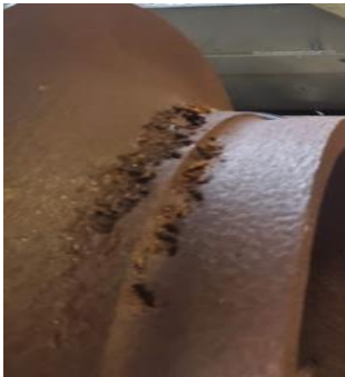
Cavitation damage on impeller shroud
